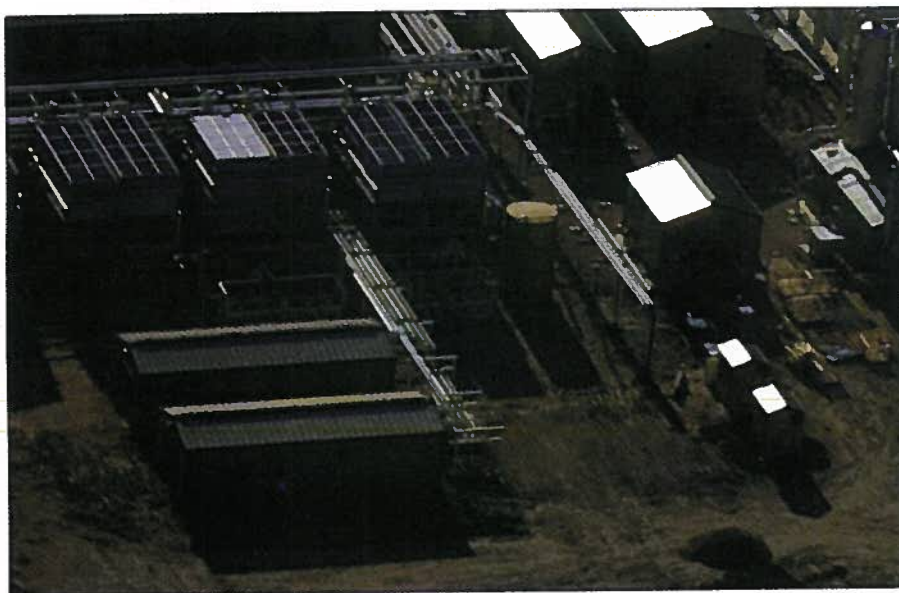
The injection pumps are in the two long buildings in the lower left. The pipe rack coming out of pump buildings goes towards the aerial compressor coolers. Two variable-frequency-drive buildings are to the right of the pump buildings. Two transformers are behind the VFD buildings. The Heatric exchangers' open skid is visible behind the pump-skid building (Fig. 1).
